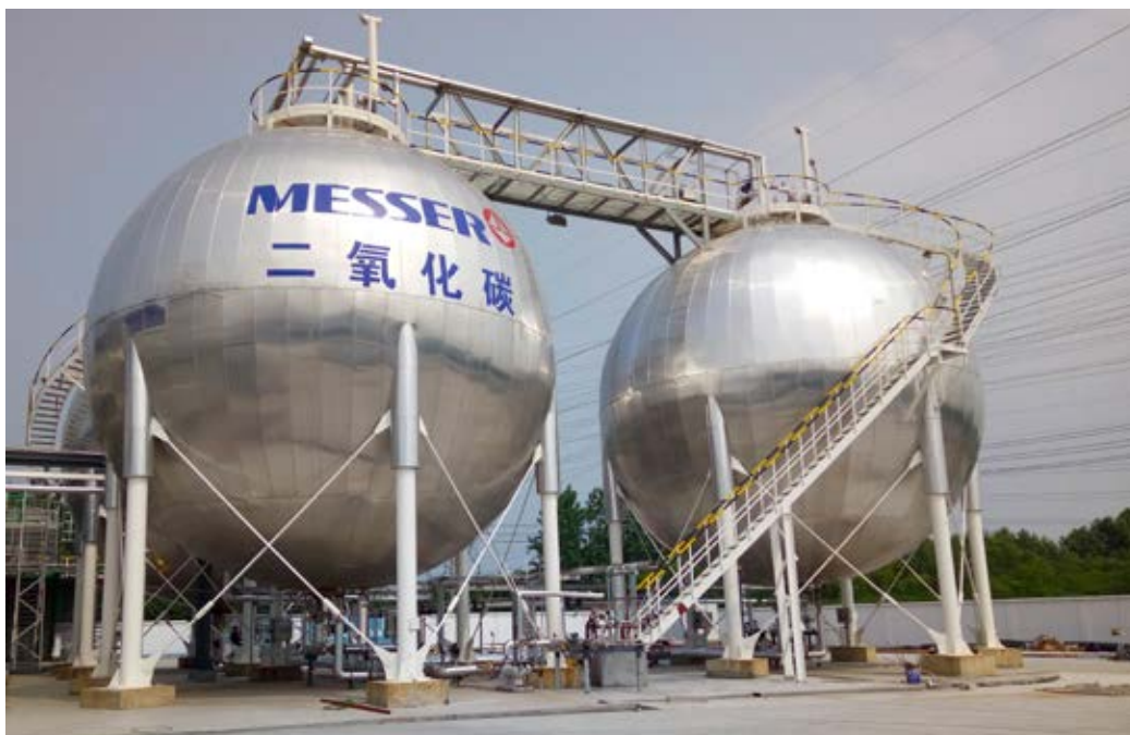
Prepared CO 2 is stored in special tanks. Customers are the food, beverage and chemical industries or agriculture.
