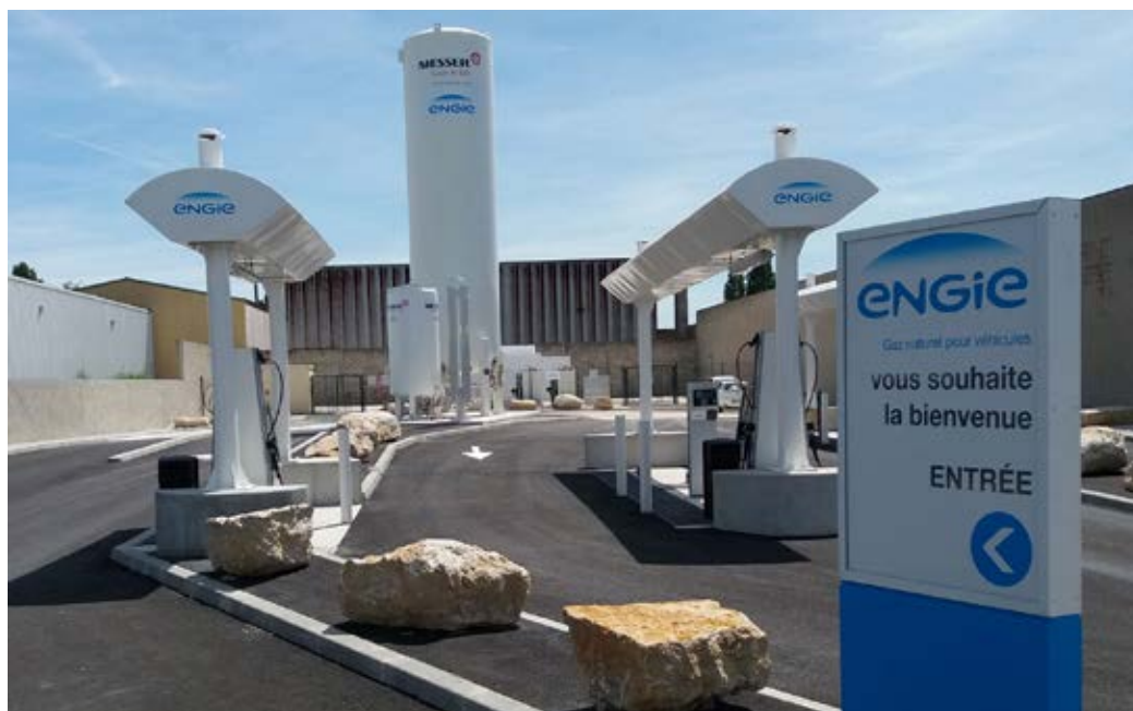
At the new ENGIE filling station, Messer operates a liquid nitrogen tank farm for trucks equipped with cryotechnical cooling units.
